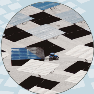
7,000 heliostats have been installed
